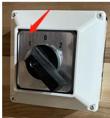
Power to stove heater
