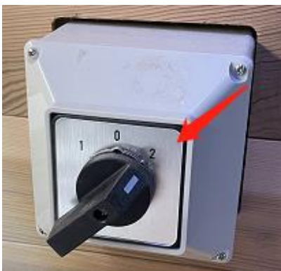
Power to Infrared heaters
