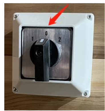
Power turned OFF
