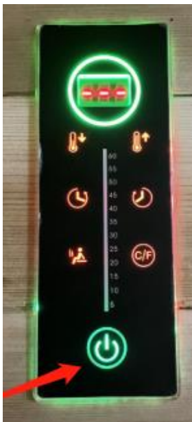
Sauna Control Panel is Illuminated
