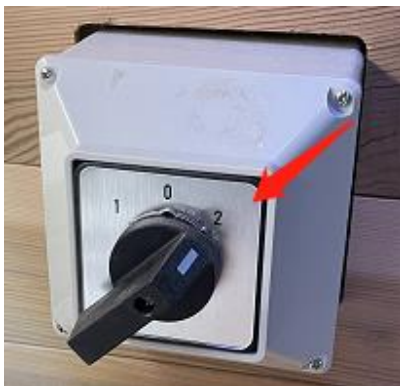
Power to Infrared heaters
