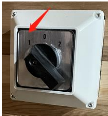
Power to stove heater
